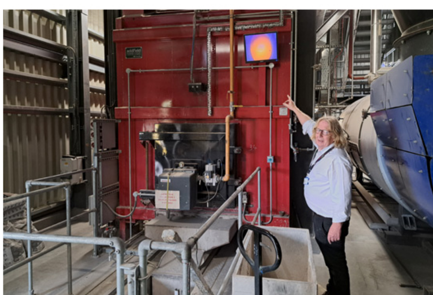
John Burrows pointing at the screen showing the inside of the incinerator
